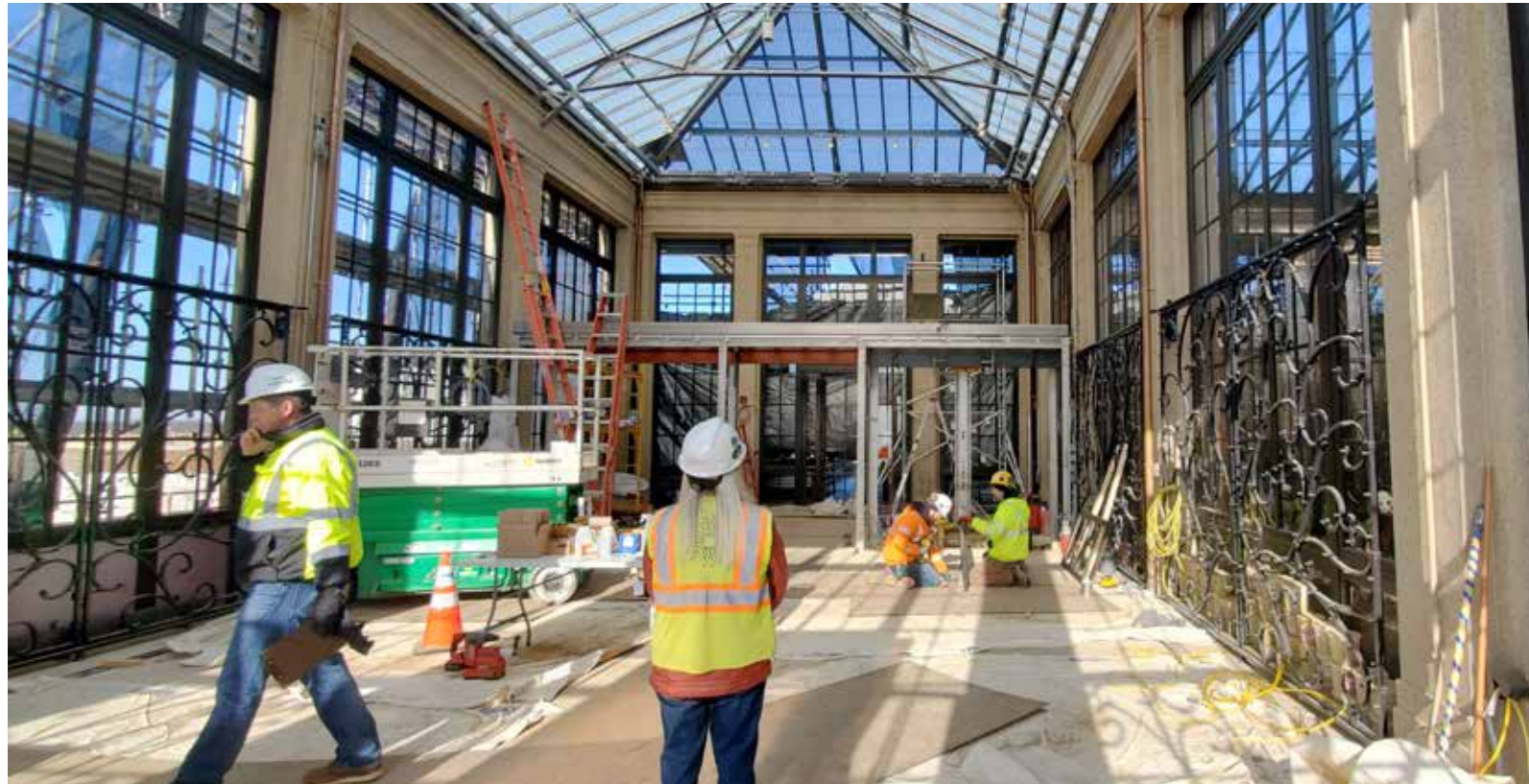
With structural issues addressed from top to bottom, work began on restoring metal windows, cases, and frames as well as the Orchid House's historic mosaic concrete. Photo courtesy of John Milner Architects, Inc.
