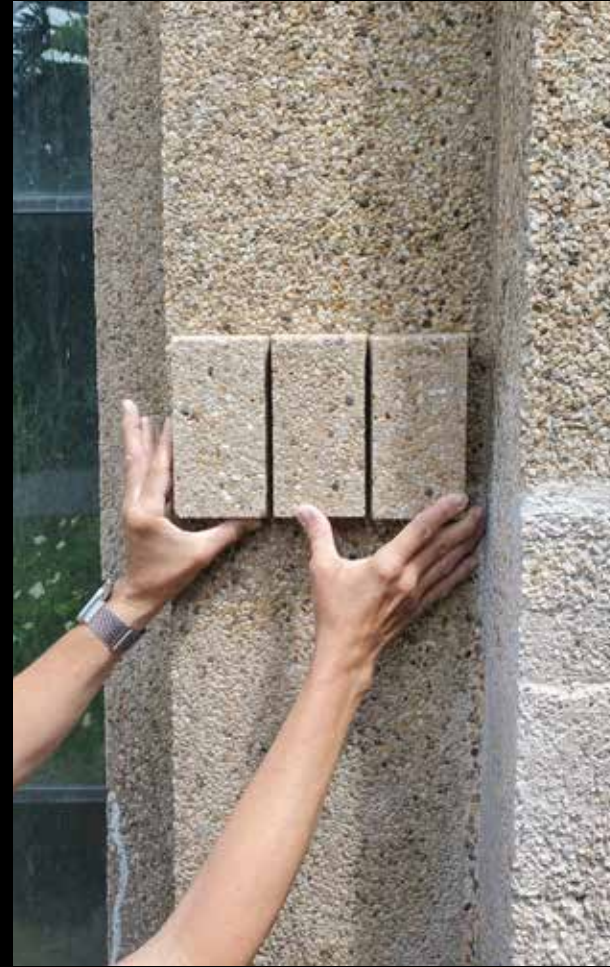
Finding the right aggregate mixture to match the existing mosaic concrete for each repair required a discerning eye. Photo courtesy of John Milner Architects, Inc.
